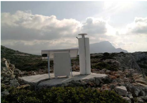
Figure 9. The SEL1 permanent GNSS site at Petra Seli, south west Crete, where water-proof box has been used for receiver and batteries housing.
