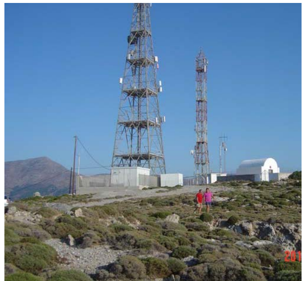
Figure 6. The KFL2 site on top of the mountains.
